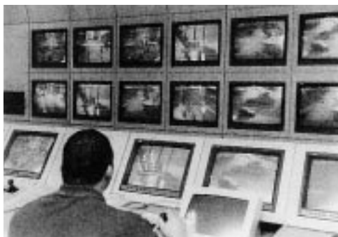
CCTV : the control room
