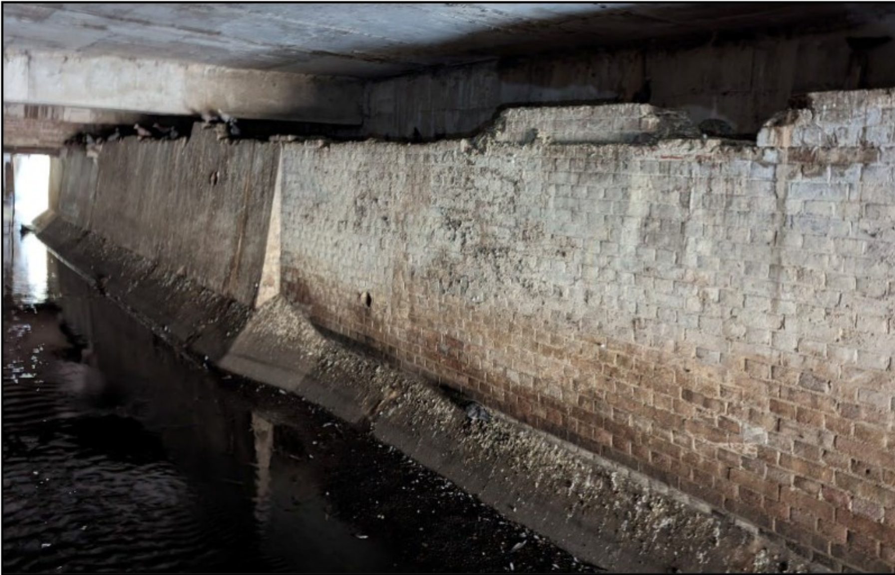
Cheapside Culvert: walls do not appear to support the concrete soffit (2023)
