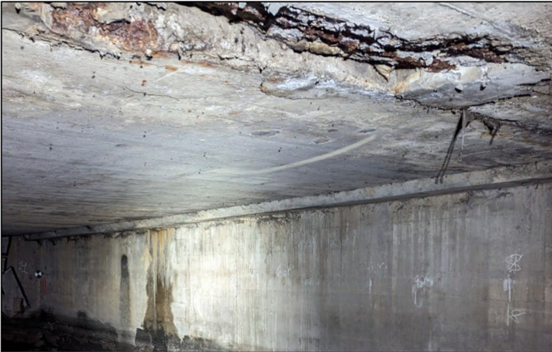
Galaxy to Hat Gardens Culvert: exposed rebar and/or steel beam (2023)
