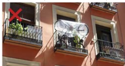
Fig. 4.3.3 Small, unuseable balconies
